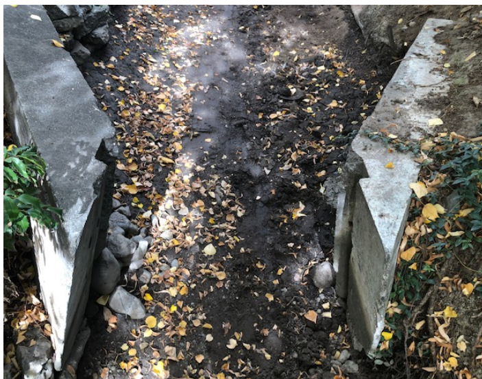
Figure 34. Overflow irrigation device in the Providence Logan Irrigation Ditch.
