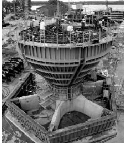
Figure 4.3.8 Gravity base foundation being constructed for Nysted Offshore Wind Farm at Rodsand, Denmark. (Courtesy of Bob Bittner, Ben C. Gerwick, Inc.)
