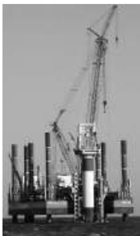
Figure 4.3.9: Monopile 50 m (165 feet) long with a 4 m (13-feet) diameter being installed at the North Hoyle Wind Farm, UK. (Courtesy of RWE)
