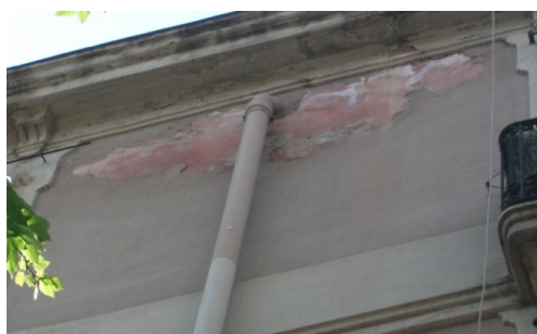
Picture 4.46: Material degradation C/ Rocafort, 161. Source: Own made.
