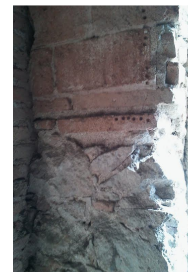
Picture 3.16: Work Mixed ashlars and brick. Consell de Cent, 377. Source: Own made.
