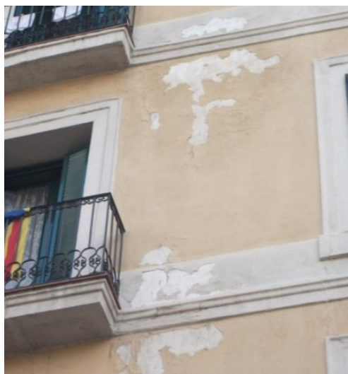
Picture 3.43: Detachment of the siding. Villaroel, 169. Source: Own made.
