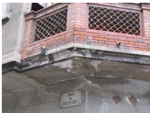
Picture 4.45: Efflorescence on de brick wall. Rocafort, 152. Source: Own made.
