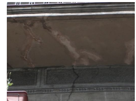
Picture 3.42: Crack on the floor slab. Paris, 169. Source: Own made.
