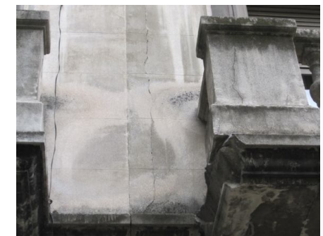
Picture 3.41: Fissures and cracks on the brick-faced. Calàbria, 94. Source: Own made.
