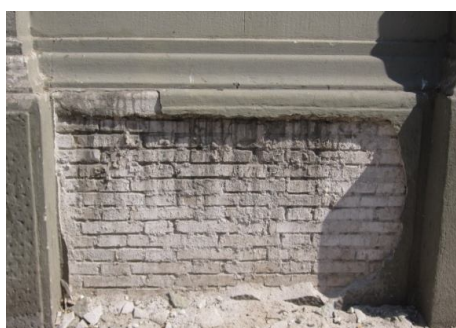
Picture 3.22: In this photo you can see low coating a section of masonry. Provenza, 164. Source: Own made.
