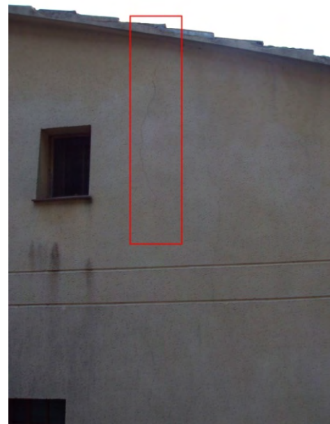
9.2.2/10. Fissura vertical, trencament del revestiment exterior
