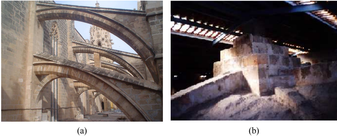
Figure 3.6: (a) Double battery of flying arches. (b) Pyramid over the key of central vault.
