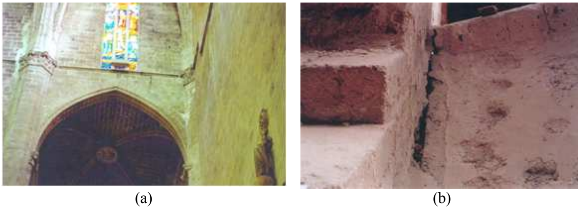
Figure 3.9: (a) Cracking in the clerestory wall. (b) Cracking by separation at the junction of central vault and the transverse arch.
