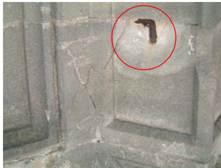
Figure 18 The rust cramp
