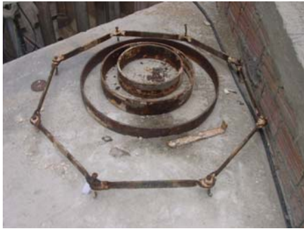
Figure 21 The corrosion of the steel components
