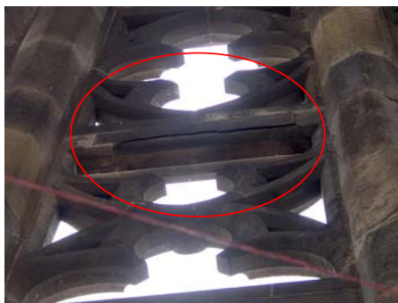
Figure 19 The crack on the pinnacle due to the metal corrosion
