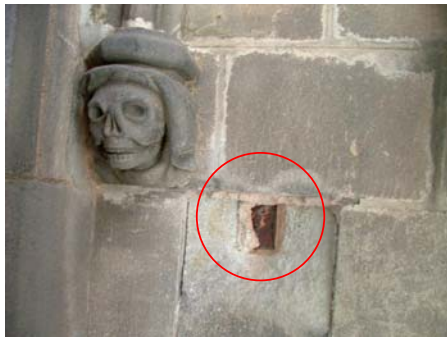
Figure 17 The rust cramp
