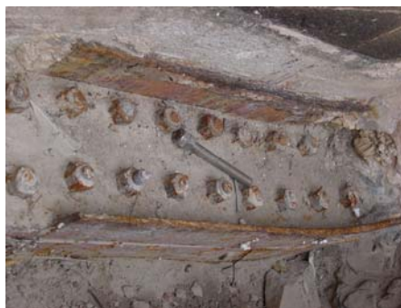
Figure 20 The corrosion of the metal elements.
