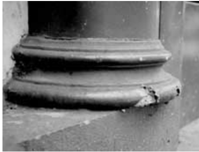
Figure 12 This lightweight fiberglass column at street level sustained damage from impact within a few years of installation. Photo: Building Conservation Associates.
