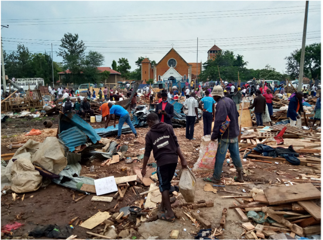
Figure 4: Demolition of the Kibuye market in Kisumu during the COVID-19 lockdown period. Traders did not get an opportunity to salvage their goods because demolition occurred during the night-time curfew. As often in such circumstances, demolition was justified on public health grounds, with construction of a new formal market planned, but with scant regard for the assets and livelihoods of the affected traders. Image credit: John Chueya (Arina Youth Group).
