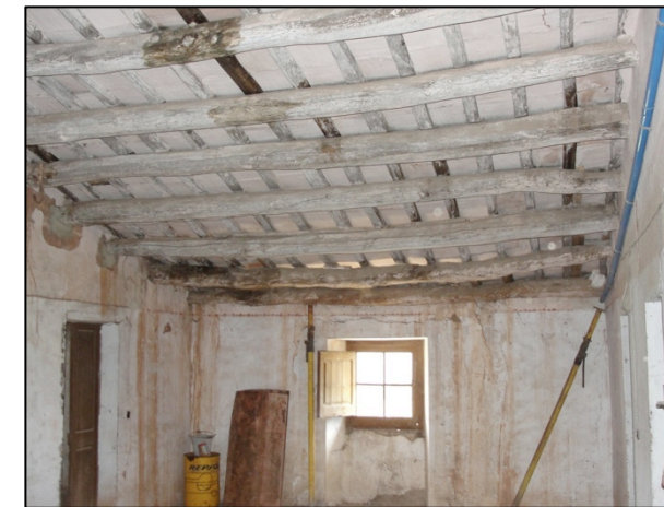
Foto 19: Bigues coberta crugia central C1-C7
