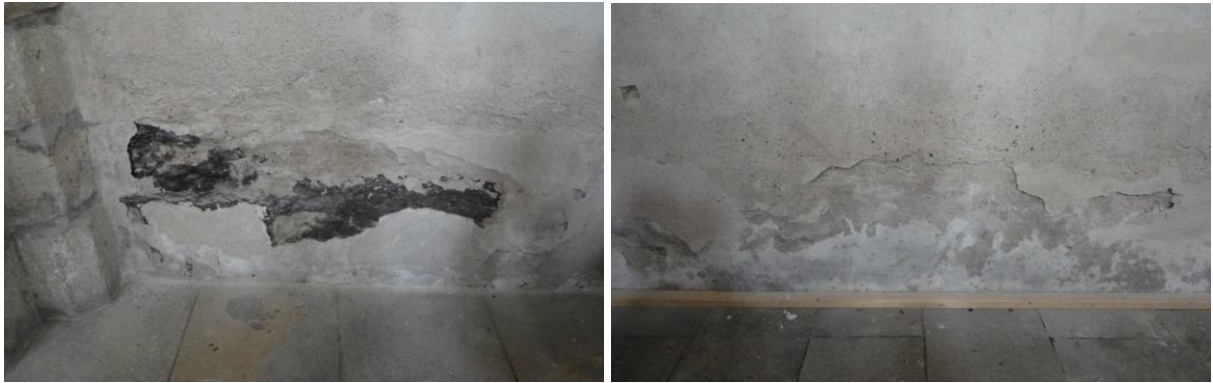
Figure 29 Damage on the interior walls
