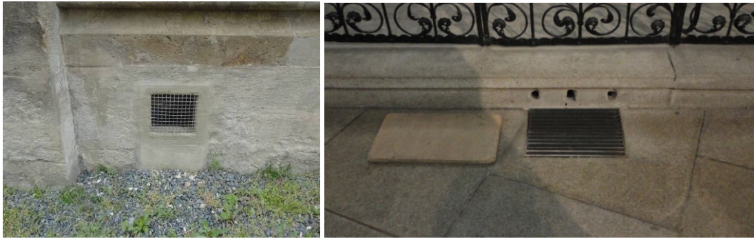
Figure 31 Grilles at the end of the vents a) from outside b) from inside
