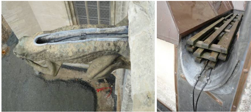
Figure 43 Heating system a) On gargoyles with slate cover b) on gutters
