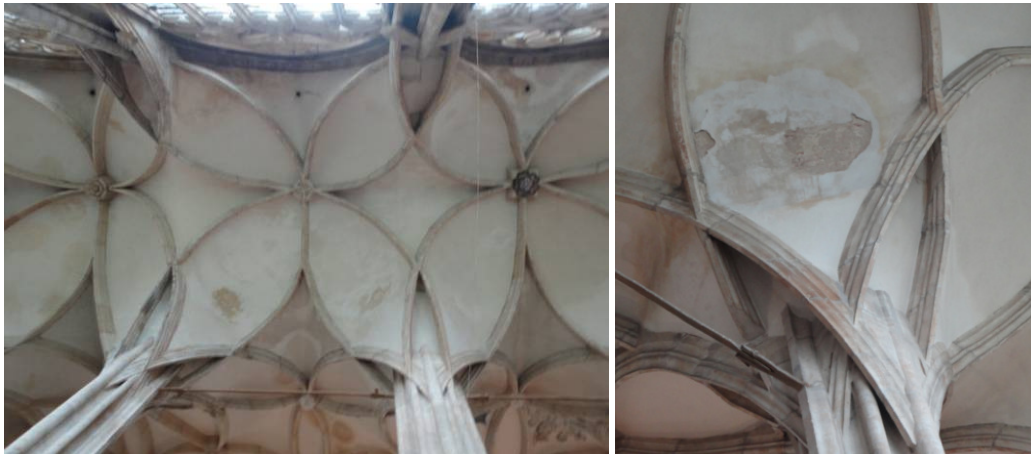
Figure 36 Decay of the vaults
