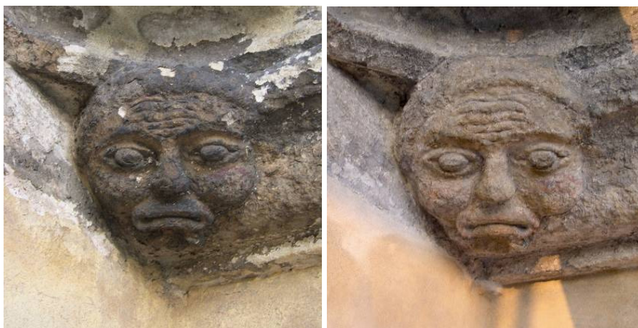
Figure 19 Mascarons a) Before restoration b) After restoration [7]
