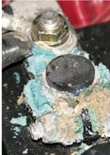
Figure 2-3: Corrosion in the external parts of the battery
