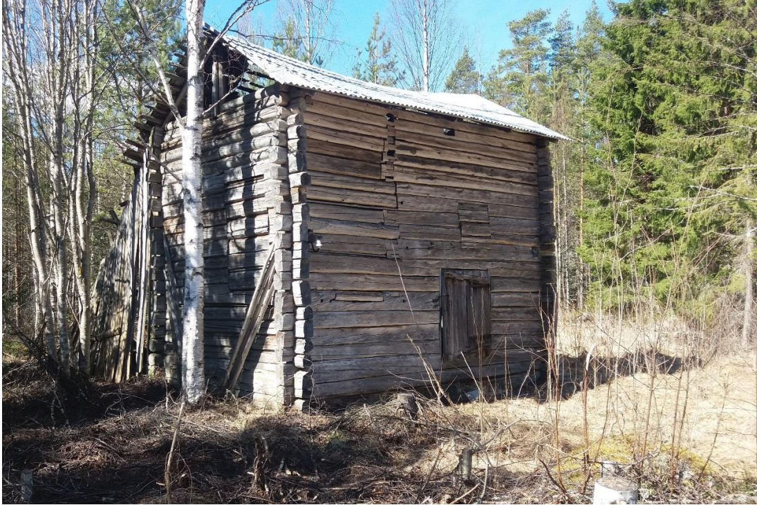
Figure 3. Reuse of logs in a granary from early 20th century, Virrat, Finland. The corner notches in the middle of the facade, which have no function there, give away the reuse. Unlike in houses, reuse was rarely camouflaged in outbuildings.
