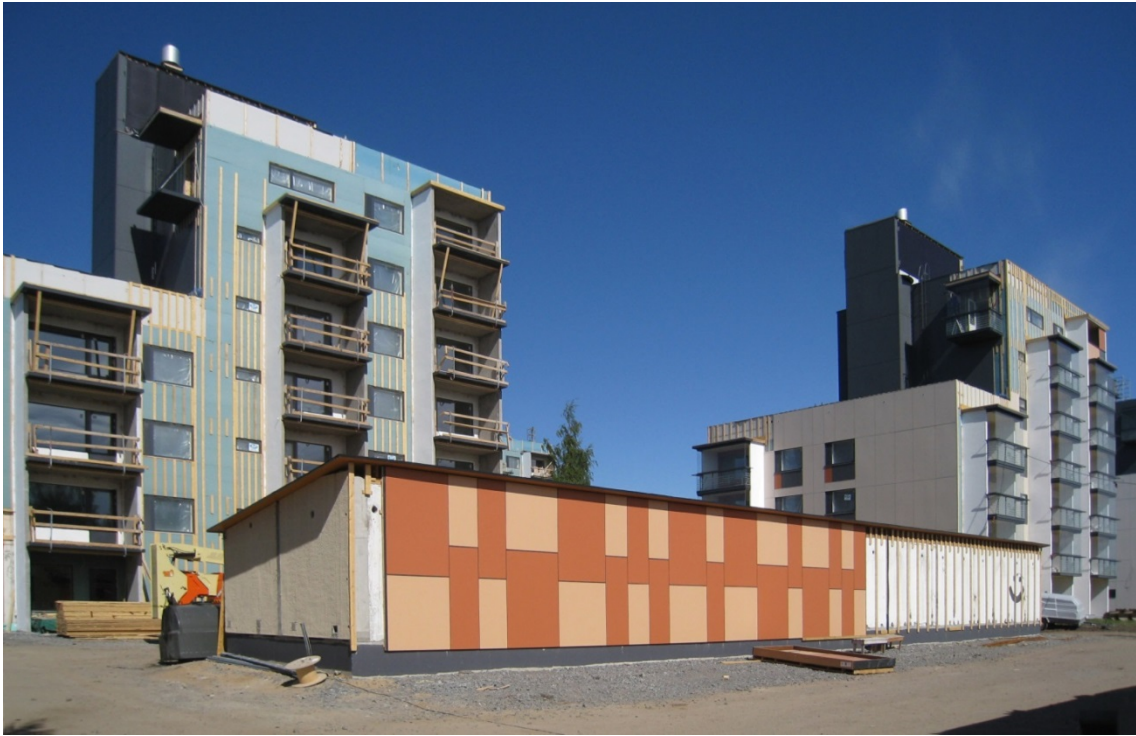
Figure 5. Construction site of Kummatti housing estate, Raahe. Partial deconstruction of apartment blocks (at the back) and reuse of panels for carports (at the front). Design by architects Harri Hagan and Petri Kontukoski. Photo in the courtesy of Petri Kontukoski.
