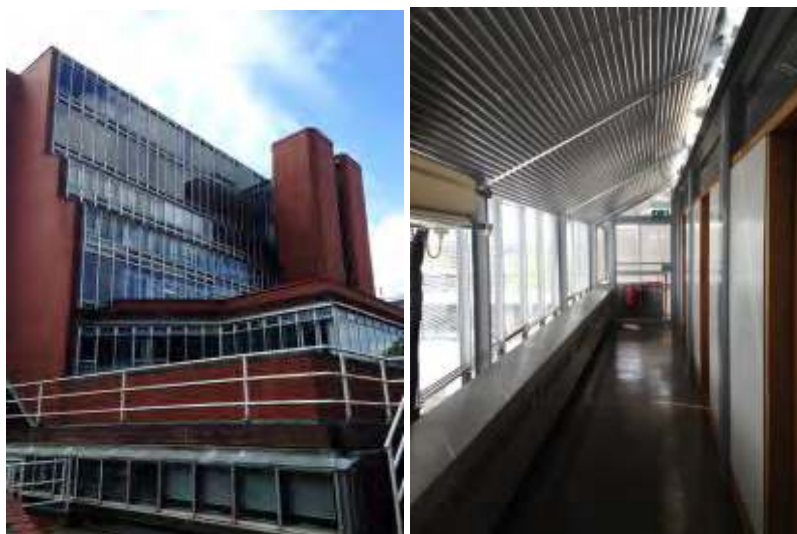
Figure 10: Excessive glazing and solar heat gain contribute to overheating
