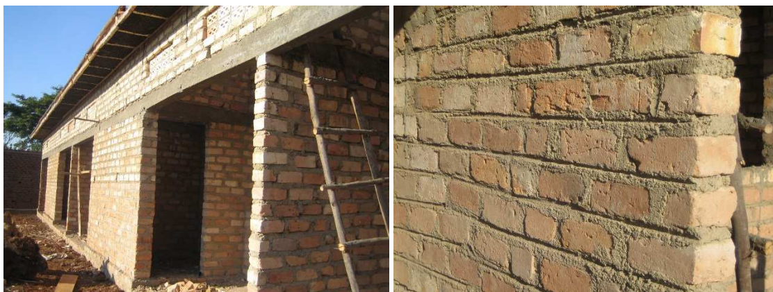
Figure 10. Excessive use of mortar due to uneven sizes/shapes of bricks. Source: The authors.
