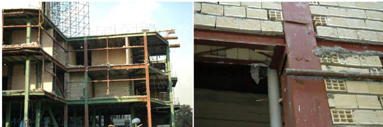
Figure 2: Low building quality in Iran.
