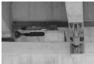
Fig. 2.26 Isolation System in the Antirion Approach Viaduct [Infanti et al , 2004]
