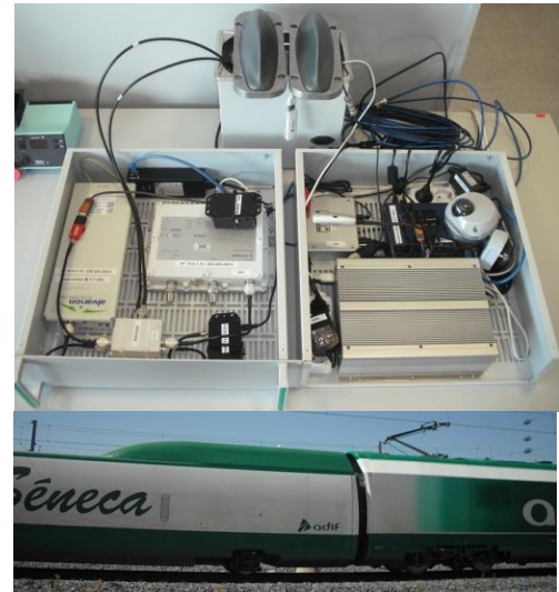
Figure 3. Wireless Communication Multiplatform installed onboard the high-speed train laboratory Seneca
