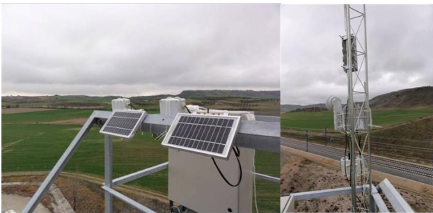
Figure 2. Autonomous nodes located in a post at 15 m of altitude next to the railway infrastructure
