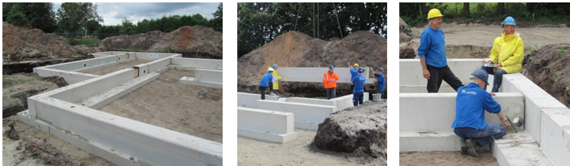
Fig.13,14,15: Prefabricated strip footings, including tie beams, can be placed on the surface or buried.
