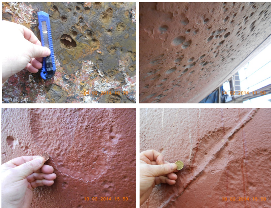
Figure 6 - Effects of severe corrosion
