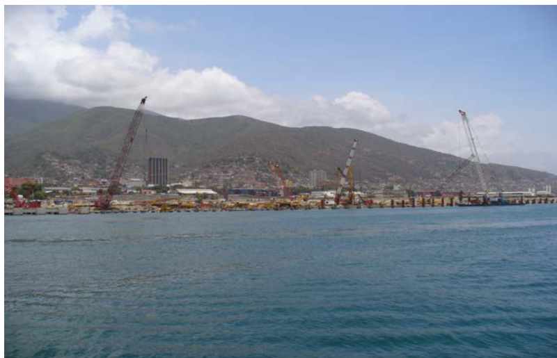
Figure 6: View of the expansion works in La Guaira port as of June 2013
