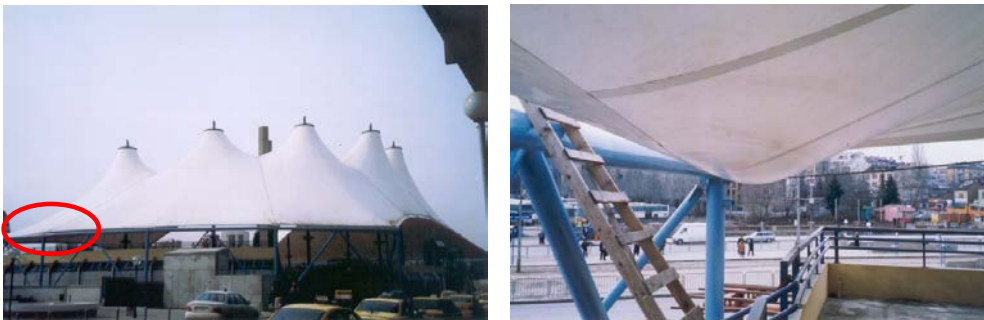
Figure 7-1 Ponding at the corner of conic structures caused by rain load in combination with rotating of the pylons (kinematics displacement) of the supporting structure [© V. Tanev]
