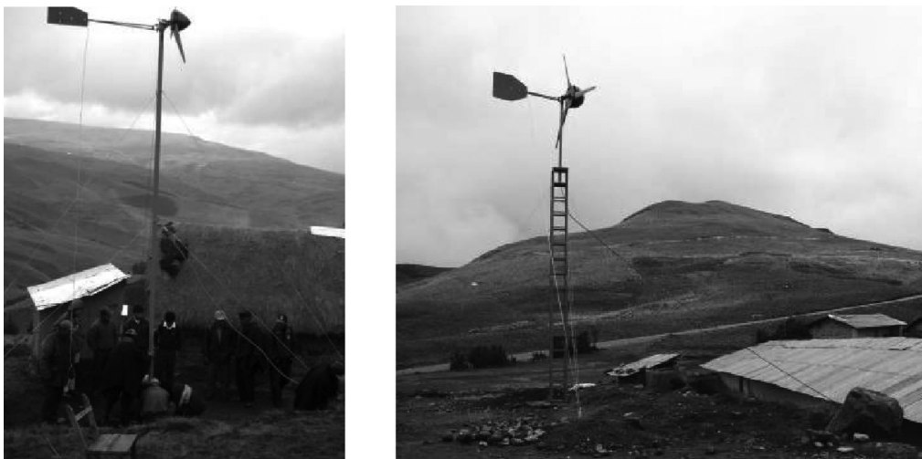
Figure 4: Installed wind generators, of 100 W (left) and 500 W (right).
