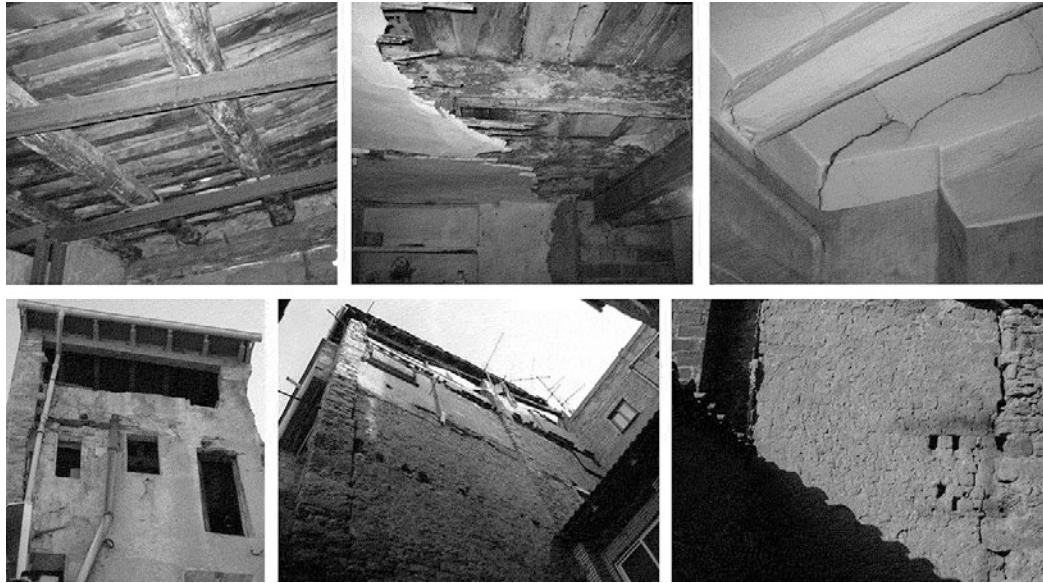
Figure 7: Existing damage and condition of the buildings.
