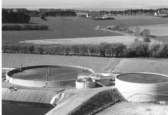
Figure 7. View of a liquid pig manure treatment plant as installed in a “typical” Brittany farm.
