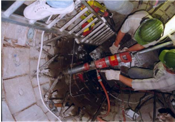
Figure 4-13: Drilling through the concrete lining of the shaft for the installation of a radial piezometer.
