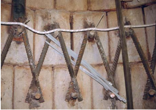
Figure 4-3: Anchorage of the two rings of blocks of the shaft lining above the future location of the seal.
