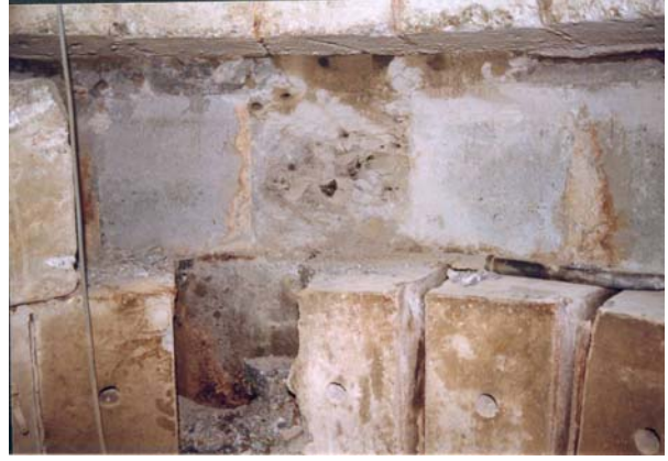
Figure 4-4: Removal of the shaft lining at the level where the seal will be installed.
