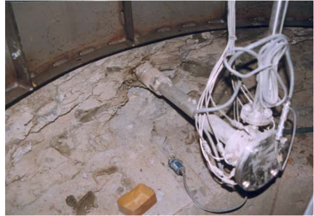
Figure 4-14: View of one of the radial piezometers, after removal of the lining of the shaft.
