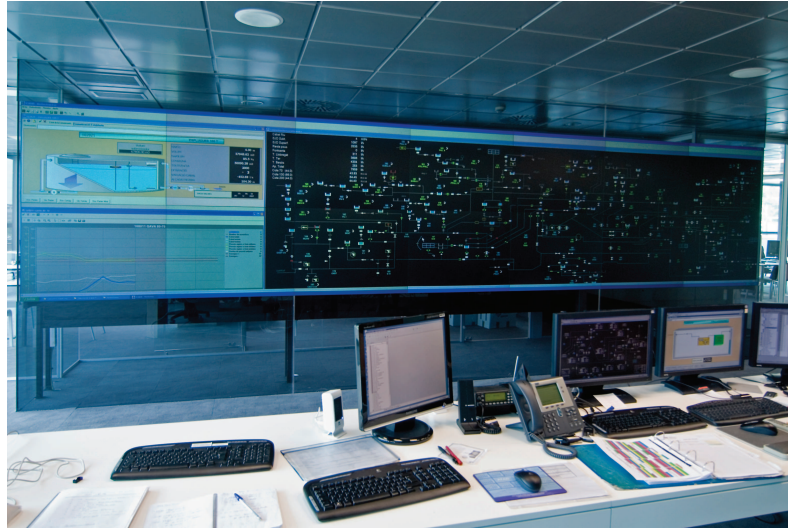
Figure 15: AGBAR Control Centre
