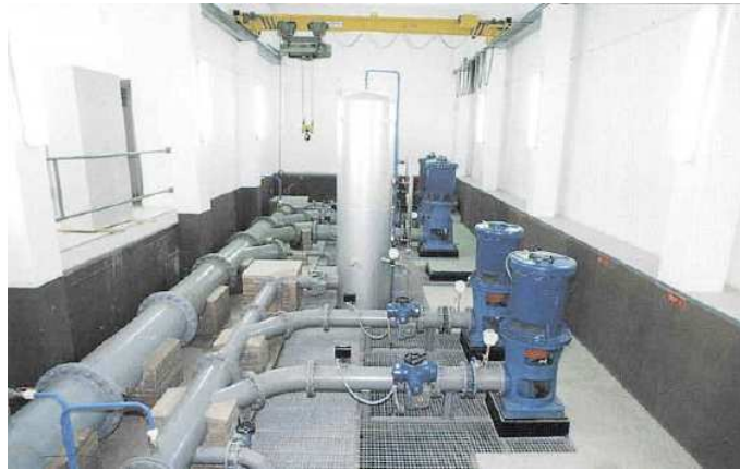
Figure 4: Drinking Water Network Pumping Station. Taken from [11]
