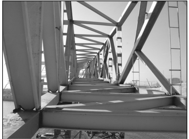
Fig. 9. The steel structure is completed. The precast concrete slab forming the platform will be supported by the floor beams
