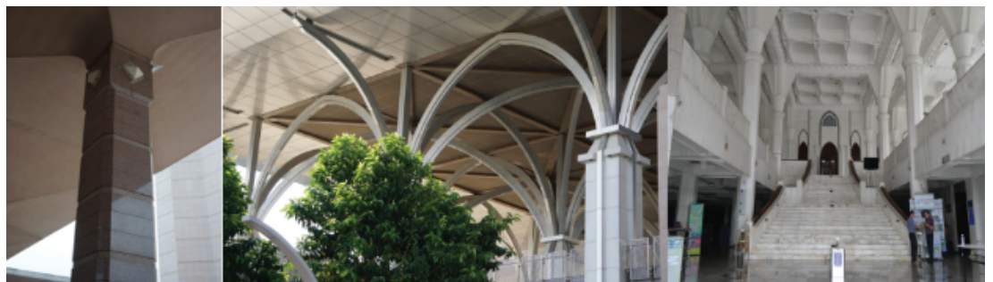
Figure 2: (Left) Concrete column of Masjid Putra, (Middle) Steel structure of Masjid Tunku Mizan Zainal Abidin (Right) Concrete columns of Masjid Wilayah Persekutuan
