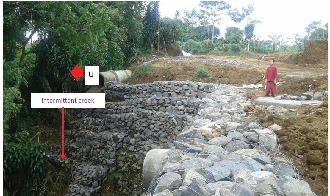
Figure 3: Gabion condition and subdrain pipe in prospective housing land (Pamungkas et.al., 2018; field work; October 2017). Soil Type at Cijeruk Area.
