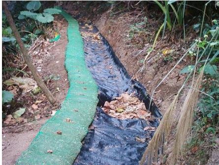
圖 7a. 邊坡坡頂回填透水材料截水 (5) Figure 7a. Water cutoff at top of slope by backfilling(5).
