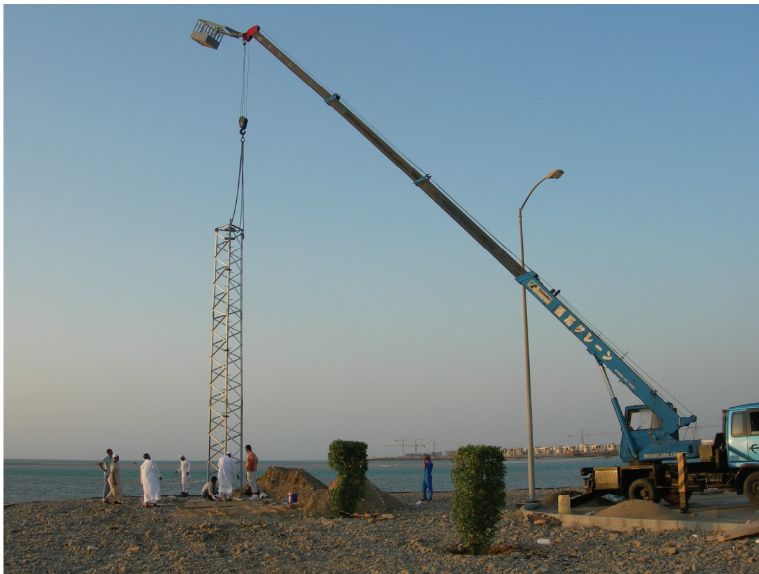
Figure VI-2: Installation of the meteorological tower on 17 October 2008 at 22°17.823'N, 39°05.567'E. Construction cranes on the KAUST campus can be seen in the distance.
