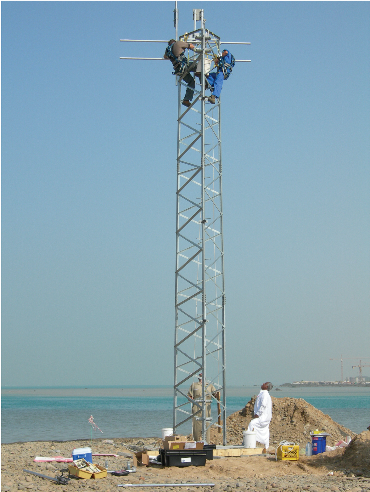
Figure VI-4: Installation of tower instruments. Farrar and Bouchard are in the tower, and Smith and the tower contractor are on the ground.
