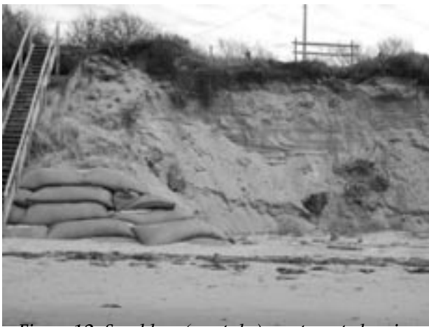
Figure 12. Sand bag (geo-tube) revetment showing end-sour
