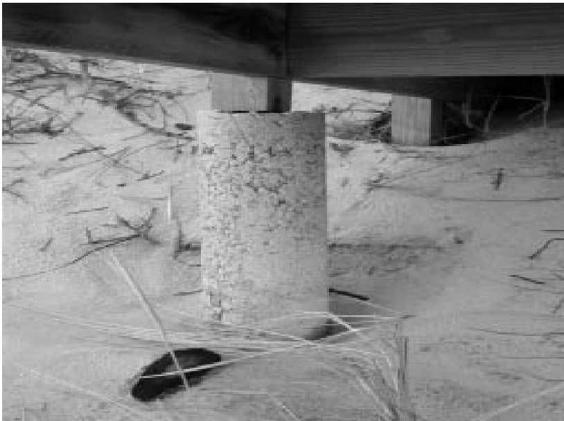
Figure 18. Wind scour around elevated dune walkway
