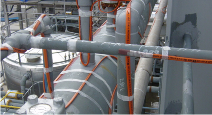
Figure 3.13: Industrial electric heat tracing (orange wires) placed on pipes and vessels, without thermal insulation [105].
