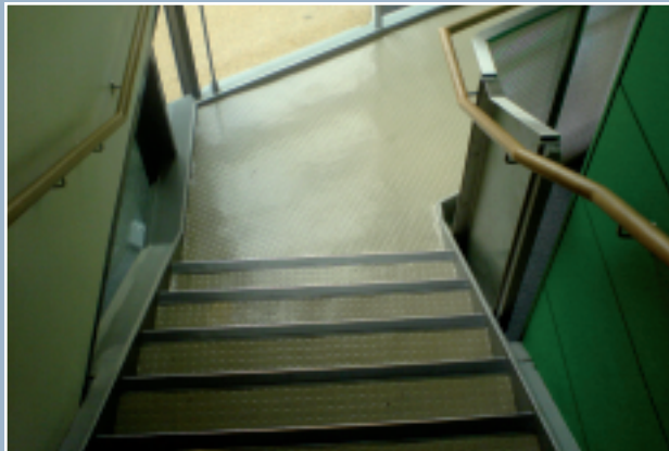
▲ Above steel staircase with studded rubber sheet finish, timber handrails and metal balustrade
