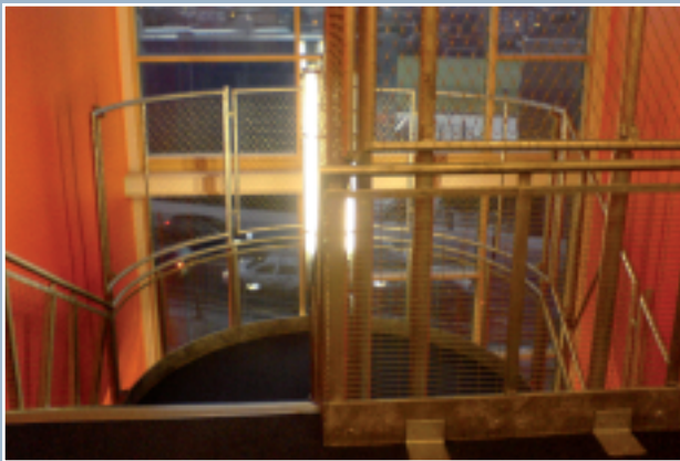
▲ Above additional safety balustrade to stairwell in galvanized metal with mesh infill
