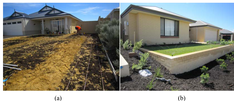
Figure 3. Photographs of garden bed preparation (a) and mulching (b) in “The Green”.
