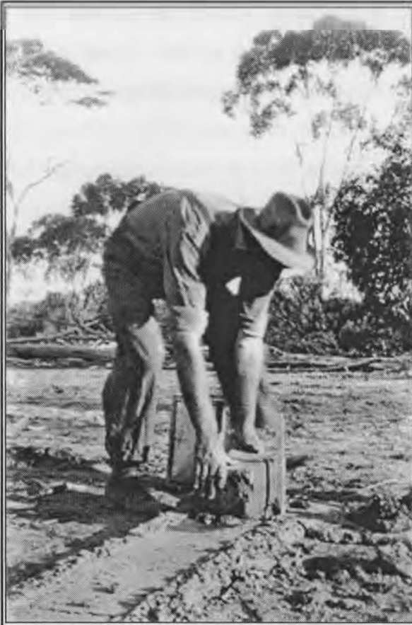
Hec laying the first mud brick for the new house at Kulja in 1929.
