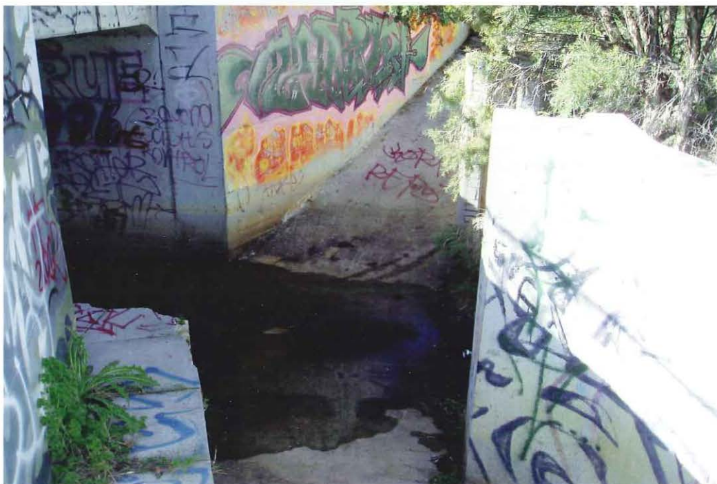
Figure 2.8 Ocean Reef Road culvert site showing the narrow channel that flow occurs through (Photo source: author).
