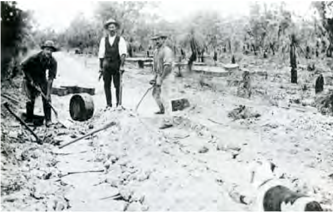
Figure 27: Jarrah wooden blocks being laid at Wanneroo Road south of Wanneroo town site in 1902.
