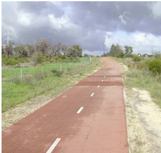
Figure 4.16: Initial portion of Route 3
