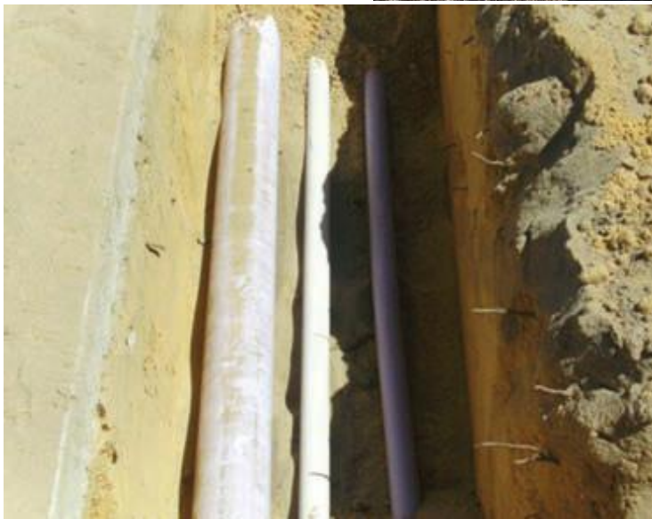
Pictures of “The Green” icon, signage, and purple pipe network for non-drinking groundwater in “The Green”, Butler
