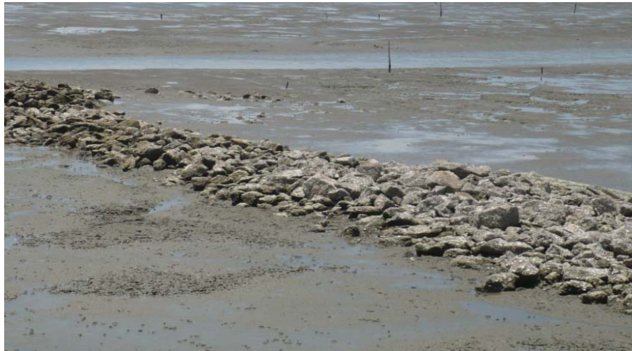
Figure 4-3. Rocks placed offshore to protect coastal area where they had fallen and collapsed.
