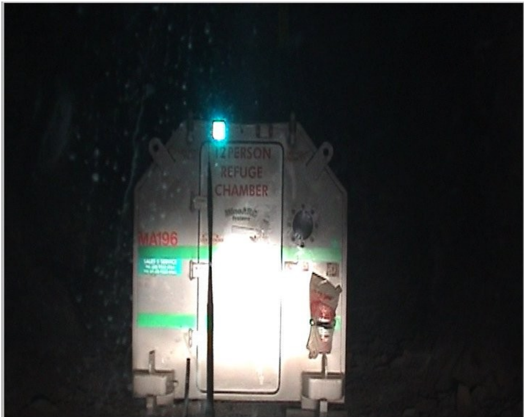
Figure 4.3. Twelve person refuge chamber in the Challenger mine
