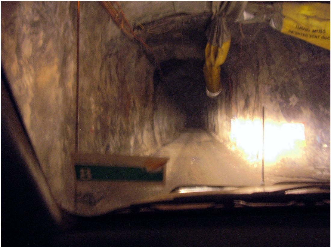
Figure 6.6. Servicing infrastructure running along the ceiling of a mine shaft in the Challenger mine
