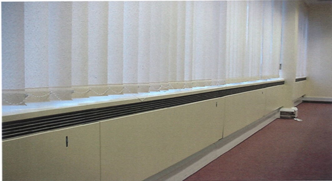
Figure (4.11): Finned-tube hot water heating system, room 302, NBB
