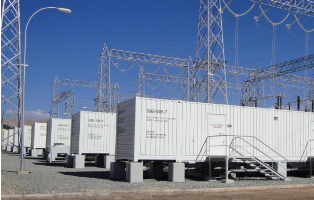
Fig. 15 The Lithium Battery Storage in Chile
