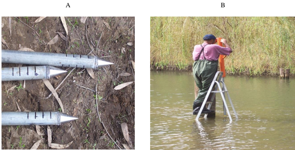
Figure 5-5. A galvanised pipe used for construction of an in-stream piezometer was designed and constructed in a local workshop at Gunnedah (A) and a fence post pusher was used to install piezometers in transects of the study area (B).
