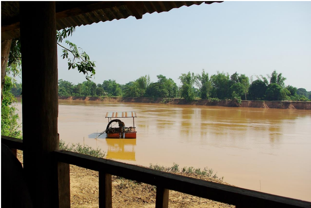
Figure 17: Severe Erosion at Sok Bo Village (author photo)
