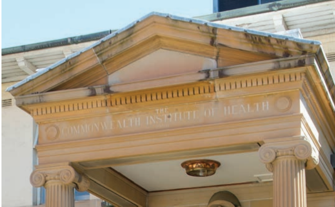
Edward Ford Building: portico above front door
