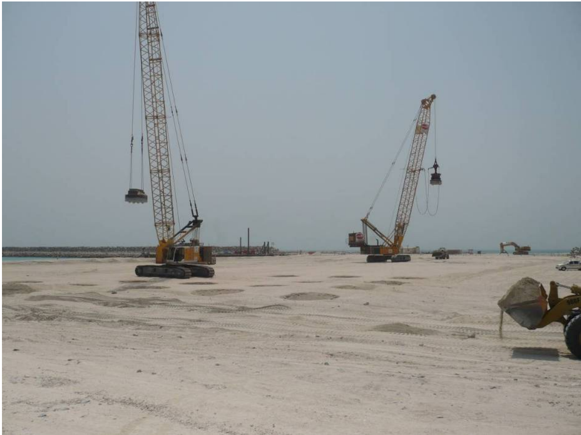
Figure 1.2. Dynamic compaction using 23 tonne and 30 tonne pounders at Port Ras Laffan, Qatar (courtesy of Menard).
