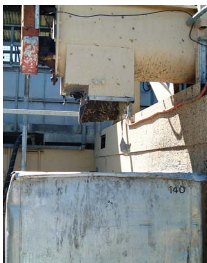
Figure 92: Corn seeper sludge pipe
