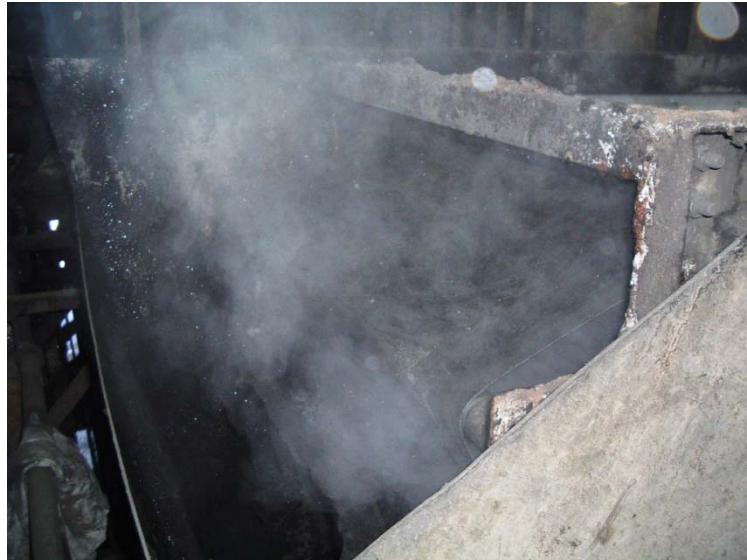
Figure 53: Number 12 boiler belt, Broadwater sugar mill
