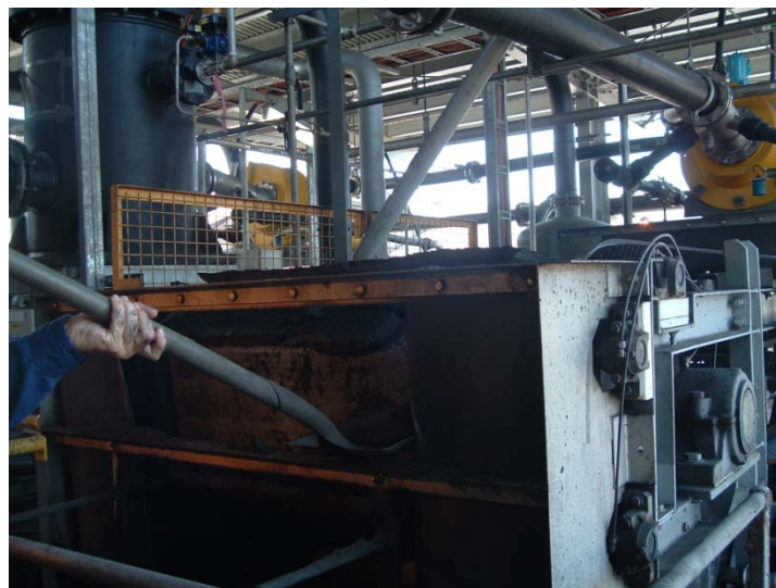
Figure 54: Number 1 boiler belt, Broadwater sugar mill
