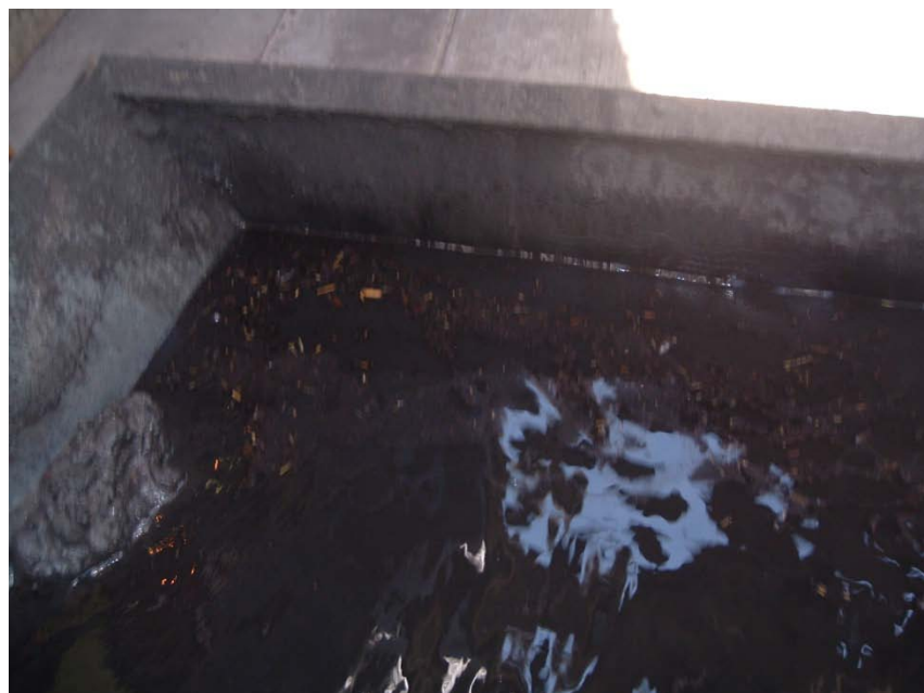
Figure 52: Number 1 boiler submerged ash hopper, Broadwater sugar mill
