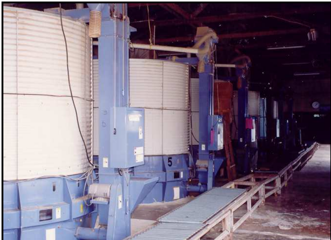
Plate 7-15 Mechanical dryers used at the Pedamaran Estate
