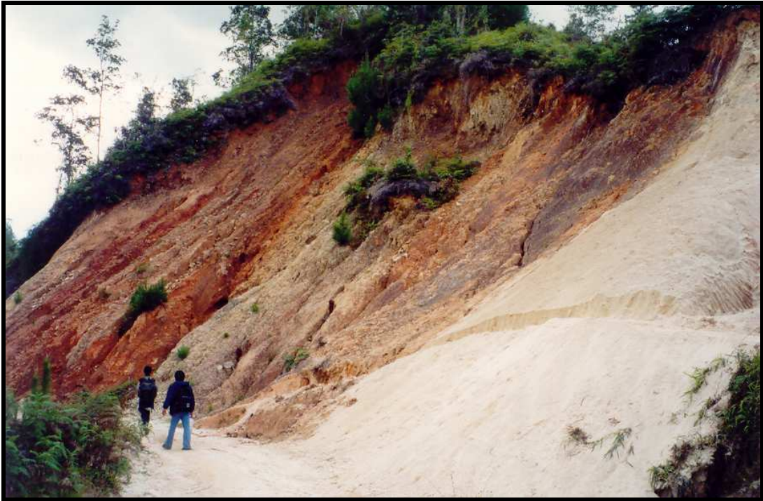
Plate 4-3 Soil erosion has continued unabated at this road cutting in Mamasa
